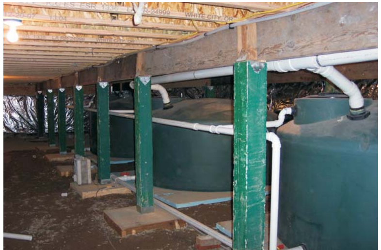
RAIN WATER COLLECTION TANKS
